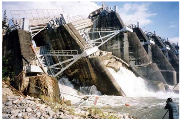
Figure 2.18. Broken spillways of ShihKang dam
