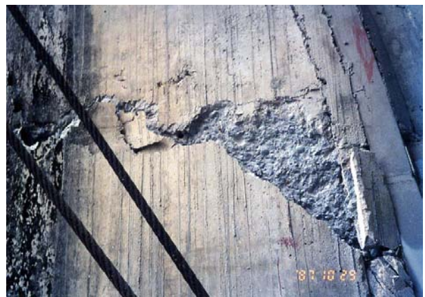
Figure 2.26. Cracks on Pier #2
