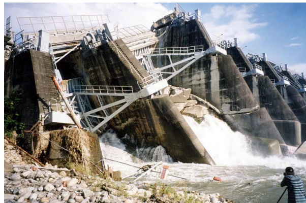
Fig. 4.9: Broken spillways of ShihKang dam
