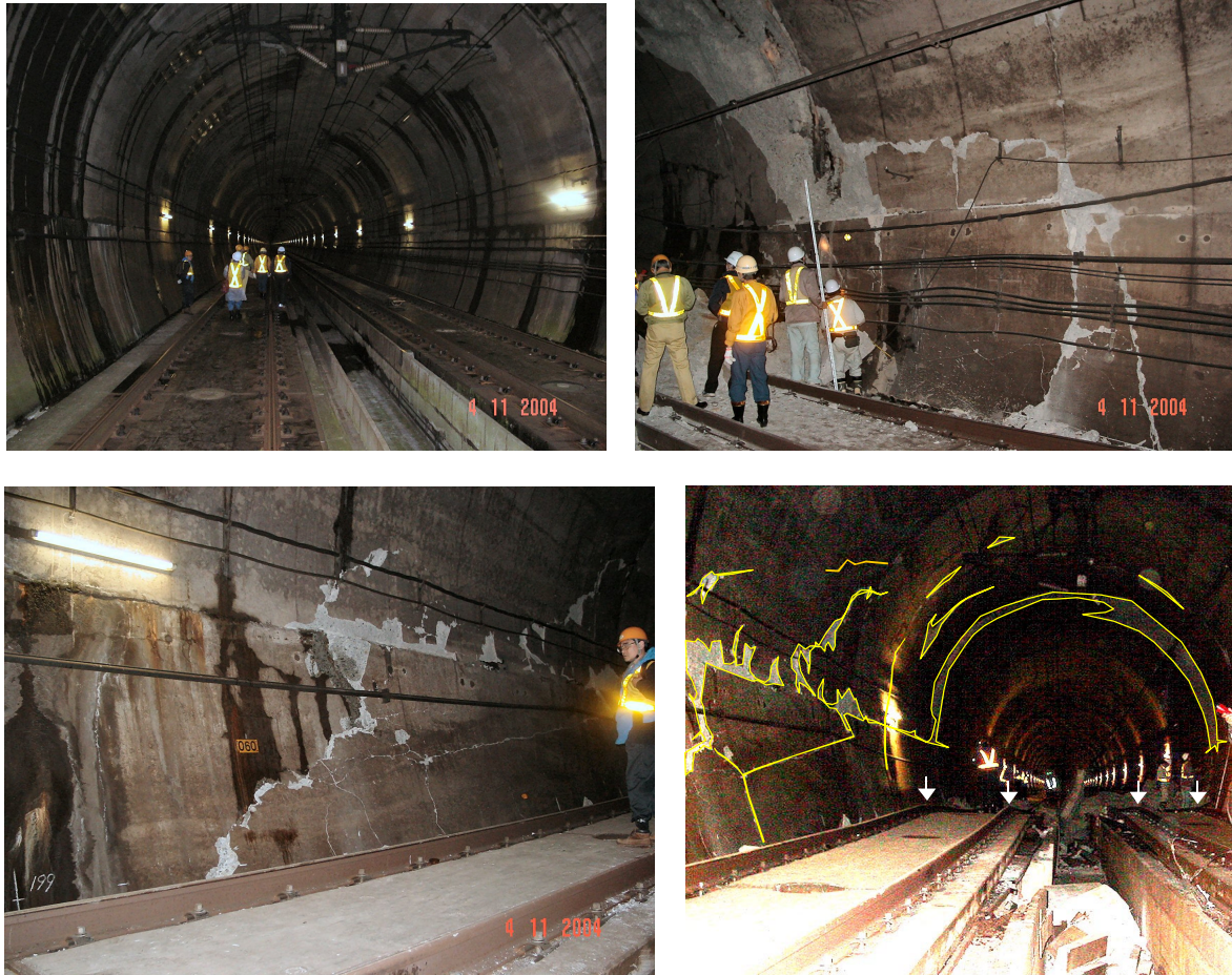
Fig. 3.20: a) Original section. b) Crack crossing the tunnel: white colored line. Top of rail is indicated by white arrows c) and d) Close up of cracks.
