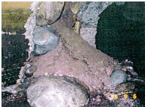
(a) Boulders squeezed into tunnel
