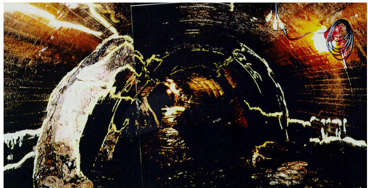
(b) Cracked tunnel
