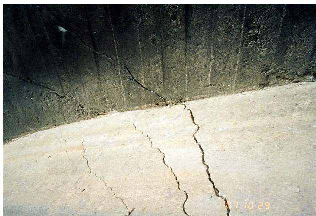
(e) Cracks extending diagonally up through Pier #10
