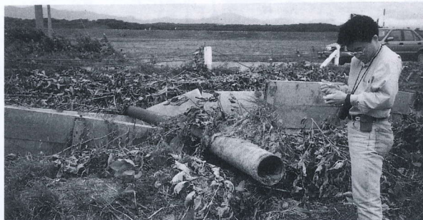
写真 4.3.5 液状化で浮き上がった水路（兜野地区） Open channel heaved up to the ground surface due to liquefaction
