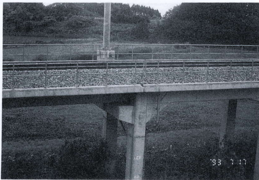
写真 4.9.1 江差線木古内川手前の大谷地区で認めた高架橋の橋桁端の圧壊 Compressive failure at the end of beam of elevated bridge, Esashi railway line, near the Kikonai river
