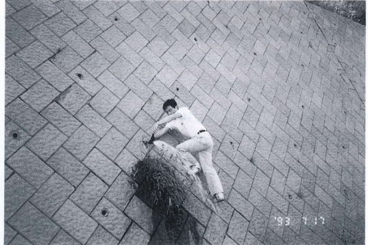
写真 4.10.7 洪積台地縁辺の擁壁の水抜き孔 (長万部) Water outlet on retaining wall (Oshamanbe town)
