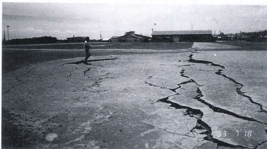
写真 4.10.2 長万部小学校校庭の亀裂 Cracks crossing the Oshamanbe elementary school grounds
