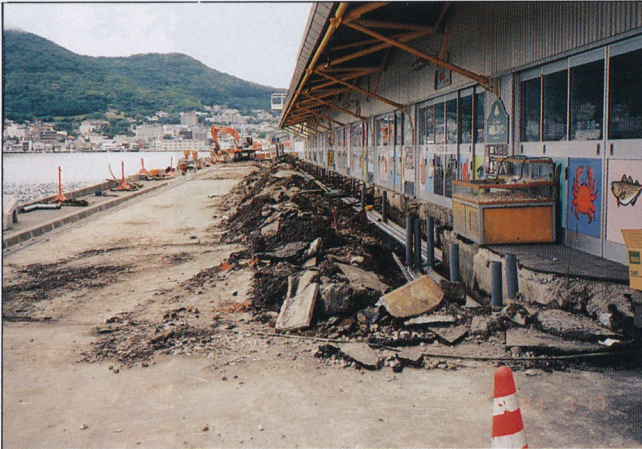
写真 4.9.3 ピアマーケット周辺の埋設管取替え工事 この付近は著しい液状化と不等沈下が発生している Repairing works of lifeline around the Pier Market. Liquefaction and uneven settlement took place all around the building
