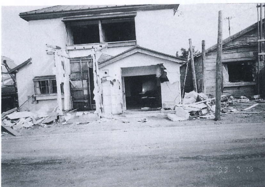
写真 4.2.6 馬場川河口左岸 民家の津波被害 (1) Houses damaged by tsunami (mouth of Baba river) (1)
