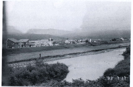
写真 4.9.2 木古内川右岸堤防の護岸の被害 Damage to riparian works, right bank of Kikonai river
