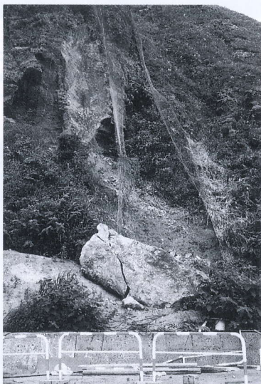
写真 4.4.5 鷹巣岬坑口付近(2) 落石と金網 Steel net preventing stone falling near the entrance of tunnel (2)
