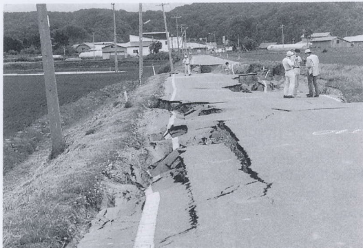
写真 4.4.22 今金町豊田の農道の被害 (1) 約 100 m に亘り沈下、破壊 Settlement and lateral spread of road (Toyoda district) (1)
