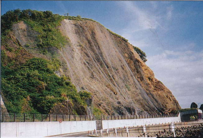
写真 4.2.10 斜面崩壊と落石防止用金網 Slope slide and steel net to prevent rock fall-related damages
