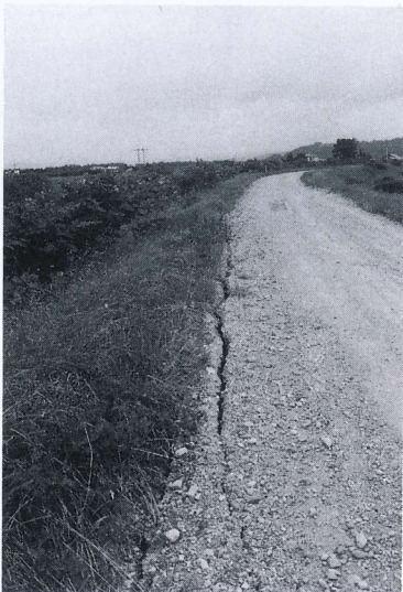
写真 4.4.17 パンケオイチャヌンペ川の堤防の被害 (2) Longitudinal crack along the slope shoulder of the left bank (Panke-oicha- nunpe river)
