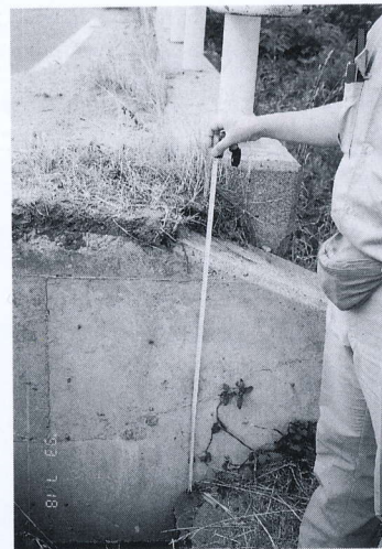
写真 4.3.20 橋取付道路の沈下 (町道兜野線) Settlement of approach road
