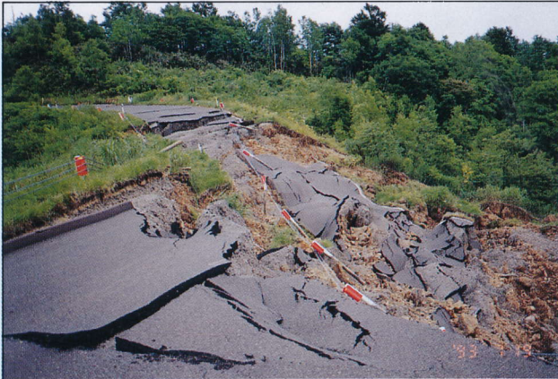
写真 4.5.2 北檜山北の町道盛土の被害 (2) Damage to road embankment (2) (Kitahiyama town)
