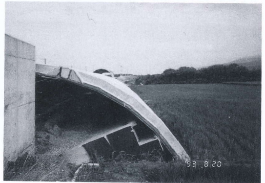
写真 4.1.14 下部工の転倒 Overturned support of the shed
