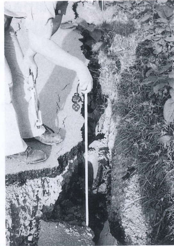
写真 4.3.19 路肩の沈下, 亀裂 (町道兜野線) Settlement and crack at road shoulder near Kabutono bridge
