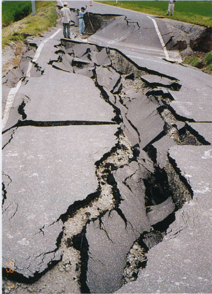
写真 4.4.23 今金町豊田の農道の被害(2) Sinking and laterel spread of road embankment (Toyoda district) (2)
