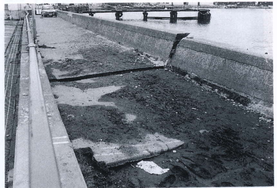
写真 4.9.7 棧橋駐車場護岸の不等沈下の液状化による噴砂 Fine sand spouted out by liquefaction and settled retaining structure(Sea Port plaza)
