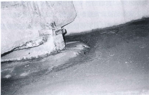
写真 4.7.1 目名川橋左岸橋台上の支承部 Cracks and movement of bridge support at the left abutment, Mena river bridge
